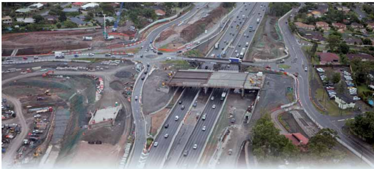
An aerial view of construction progressing on the new Loganlea Road interchange.
